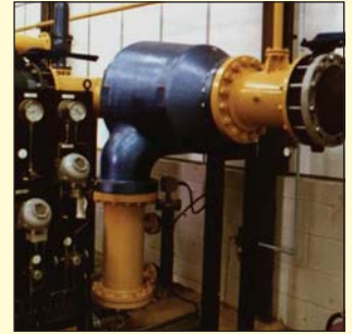
12" KSS Cyclone & Reservoir
