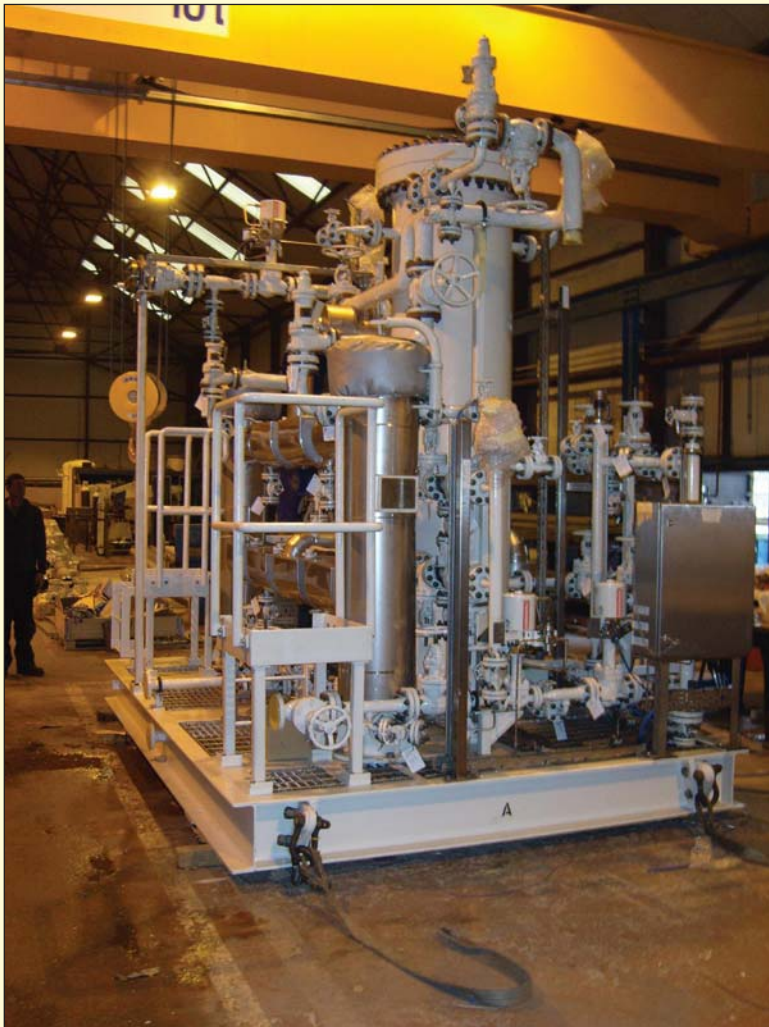
Fuel Gas Conditioning Skid
