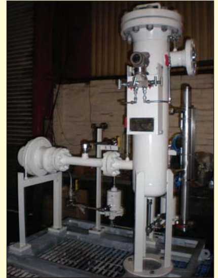
Fuel Gas Separation Filtration Skid for Gas Turbine
