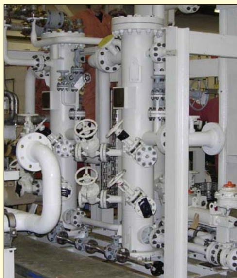
Duplex Coalescer Filter (Duty / Standby) Arrangement Gas Treatment Skid
